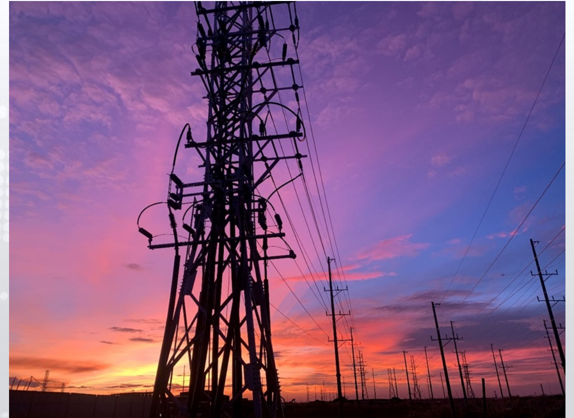
The completed power collection system
