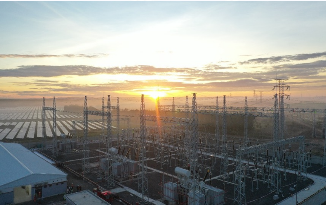
The completed step-up substation
